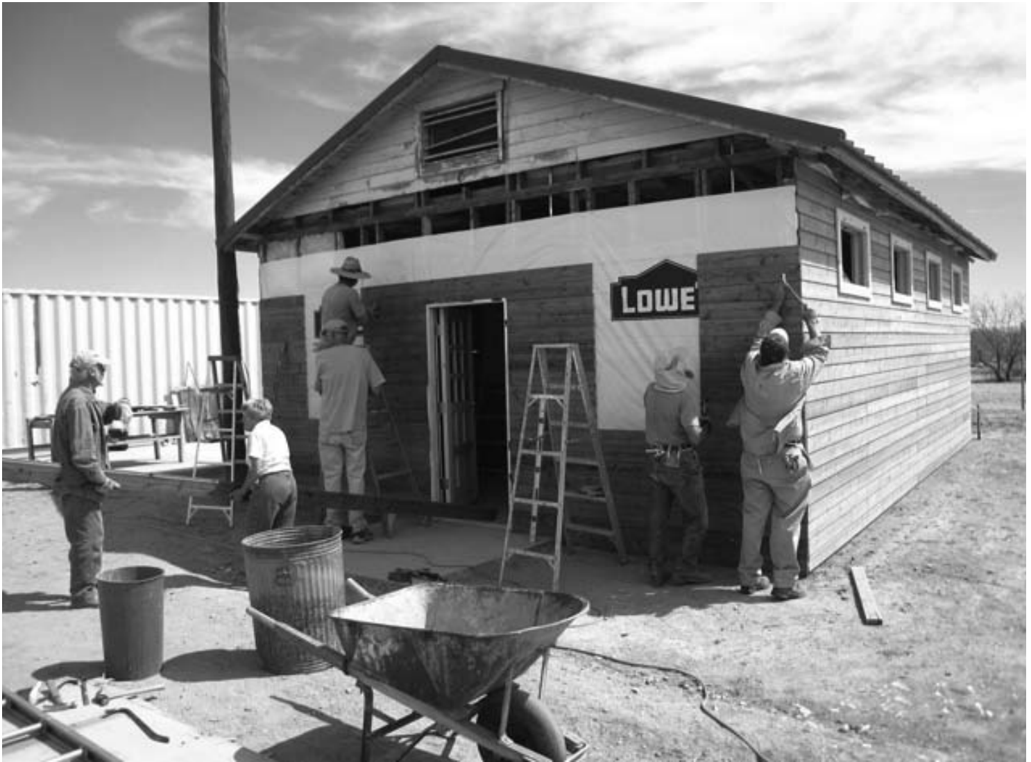
SWAT members are busy installing new exterior siding around the new front door of the Toltec Schoolhouse
