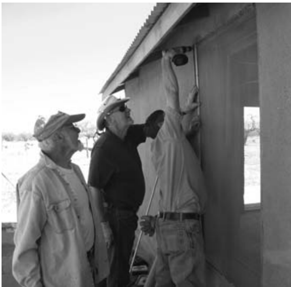
Ed Mack, Wilson Allen, and Jerry Howard install screens on the Verdugo schoolhouse building.
